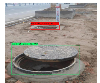
Intelligent identification of tube well risks (missing, warped, damaged)
